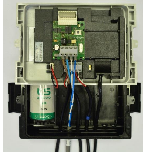
Picture 5.6 - Example of correctly wired module
